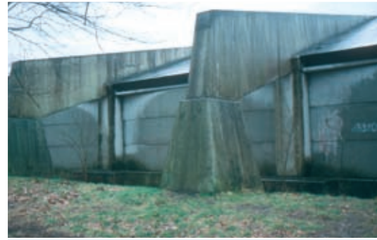
This large concrete barrier that cantilevers over the hard shoulder of the A28 motorway at Zeist in the Netherlands protects the adjacent housing estate from the traffic noise.
