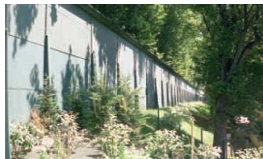
Painted green on the traffic side to match the plane trees, this precast barrier near Paris incorporates sound absorptive concrete and an anti-diffraction coping.
